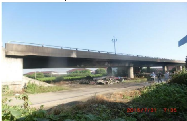
Fig. 4. Fire-damaged S12 bridge.
