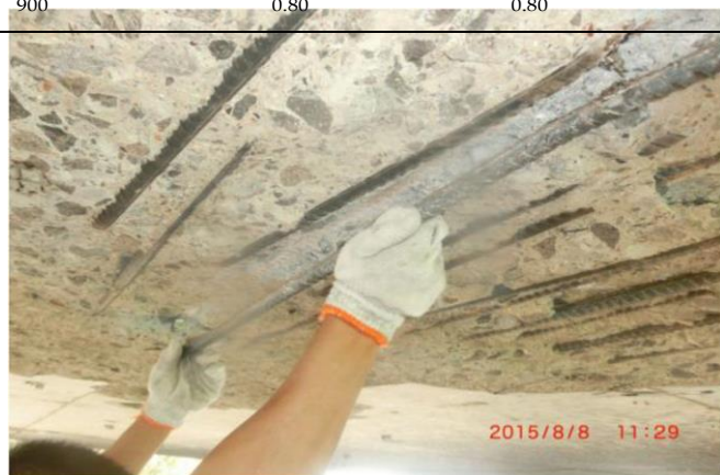
Fig. 11. Bar sample from the soffit.
