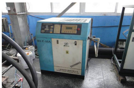
Figure 4 Bolaite BLT15A gas compressor.
