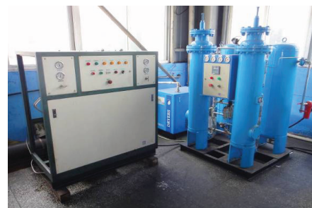
Figure 3 RIDE RDN nitrogen generator.
