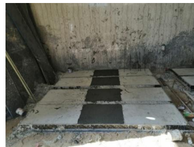
(e) Installing the steel and casting the SHCC layer and finishing the surface
