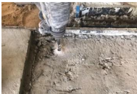
(b) Using the drill to make a concrete hole to install the dowels then cleaning the hole from dust by blower
