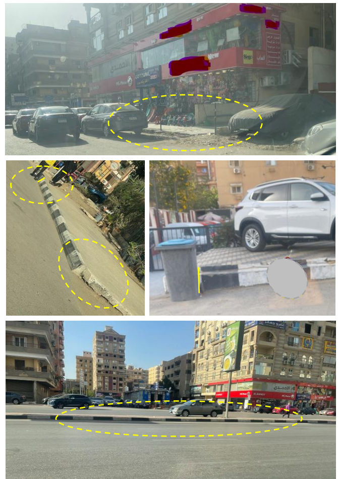
Figure 34. a), b), c), & d) Sidewalks and curbs various photos showing their current state, height, finishes, and unauthorized occupations marked using yellow shapes [17] (26/4/2023).
