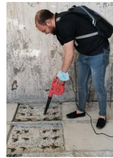
(d) Cleaning the area from dust by blower and paint the surface with epoxy.
