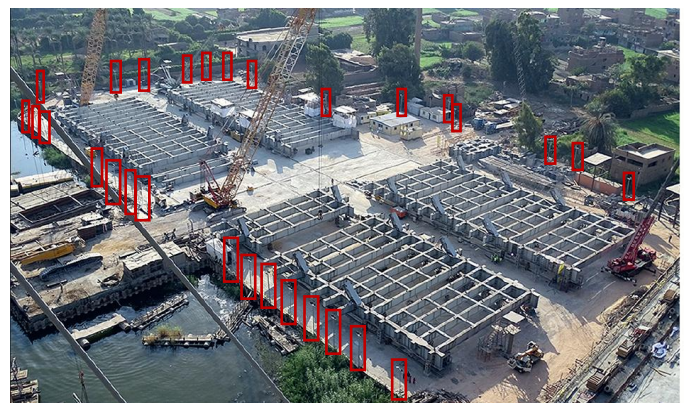
Fig. 2. Adopted from Yu and Chen [23], shows the preassembly yard, which is divided into four identical quarters, each quarter has four segments to be assembled. And also presents the allocation of the used luminaires in the preassembly yard, adopted by project administration.
