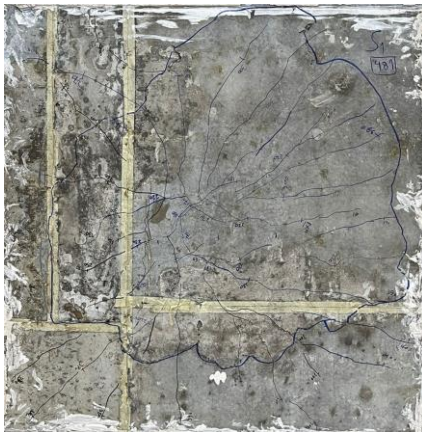
(i) Crack patterns of S9
