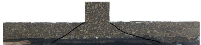
(a) Crack patterns of S1
