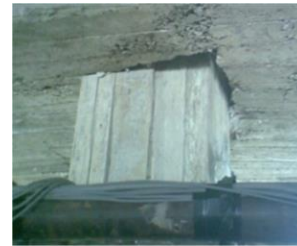
Figure 1. Punching shear failure.
