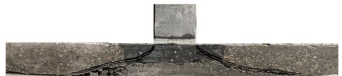
(c) Crack patterns of S3
