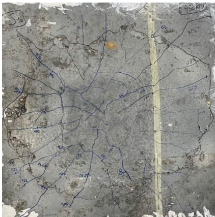
(j) Crack patterns of S10
