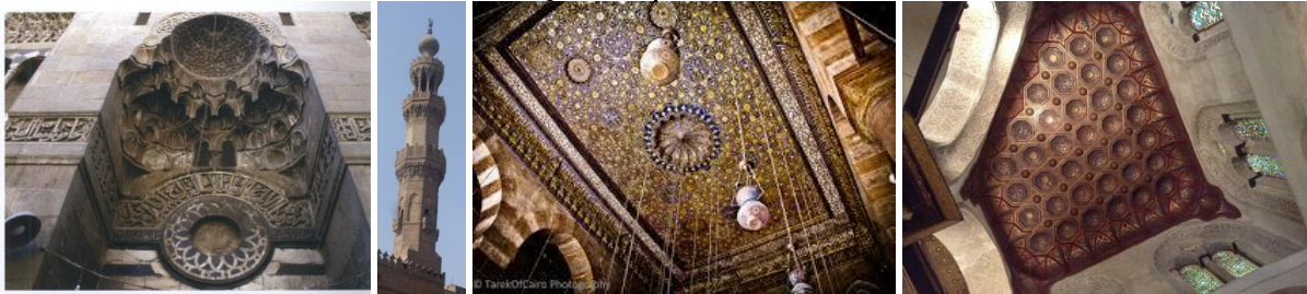
Figure (20): Different structural connection elements in Mamluk religious buildings, left to right: 1- Muqarnas in the portal of Ahmad al-Mihmandar Mosque, 2- Shoulders in the minaret of Qadi Zayn al Din Yahya Madrasa, 3,4- Wood ceilings: (Qibla Iwan in complex of Sultan al-Ghuri, the Mausoleum in Madrasa of Sultan Qala'un. [Author]
