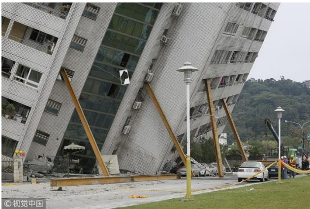
Figure 7. Differential vertical displacement failure of a structure in Taiwan Earthquake, 2018 (Lin et al., 2020).
